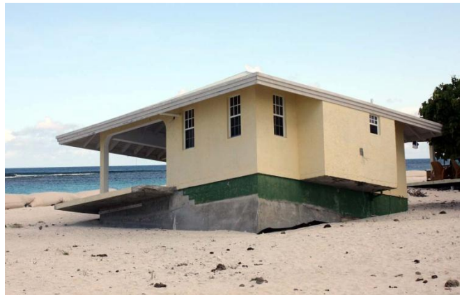
Damaged beach villa on Anegada, BVI. Sandbags trying to support beach nourishment are visible (photo: Ilan Kelman).
